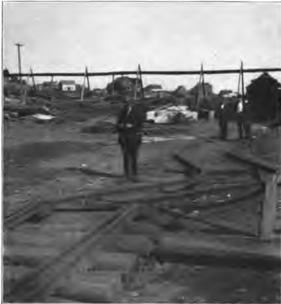
ATLANTIC MINE. N. 2.—Effect of Compression on Track Nearly Over Outcrop of Lode. Parallel Track Shown in Plate 1, and Southwesterly From It.
